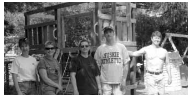
Volunteers from PotashCorp complete their Day of Caring™ project, a new play structure at the YMCA Sutherland Child Care Centre.
